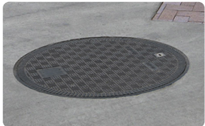
Underground Drainage System
